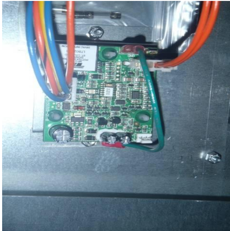
Low Water Cut Off with Ground Wire
