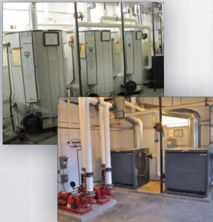
Hospital mechanical room before
