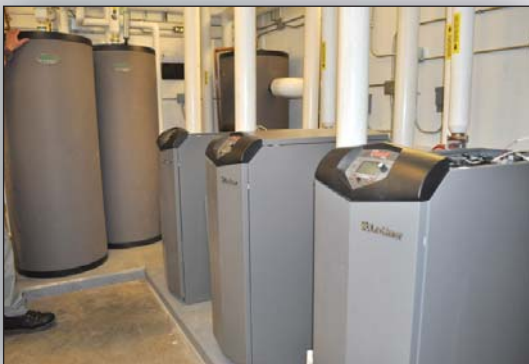
Hospital mechanical room after
