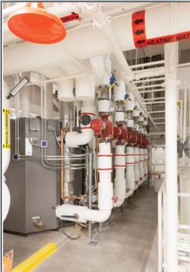
Six Crest Boilers Installed in Main Heating Plant
