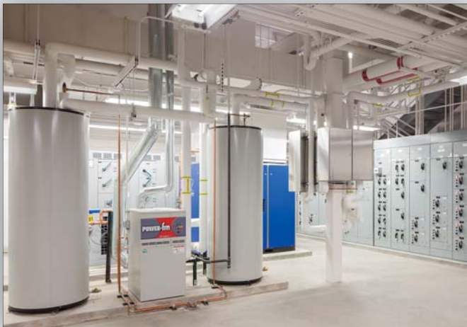
Two Power-Fin® Water Heaters Installed for Domestic Water Back-Up System, Along with Two Lock-Temp® Storage Tanks
