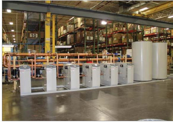
Six (6) AWN801PM with Two (2) RGA432 Storage Tanks
